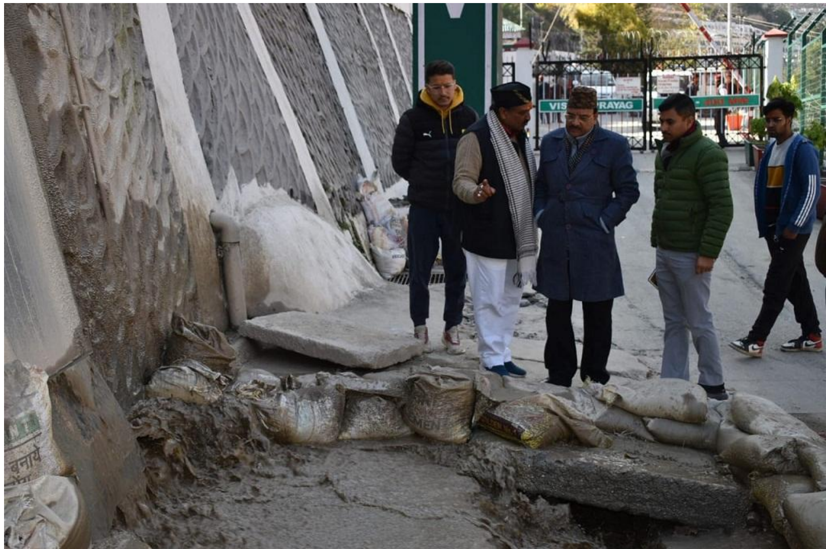
▣ The sinking town of Joshimath has been witnessing panic and anger as locals protest the cracks in the area. Photo: Twitter/ DM Chamoli.
